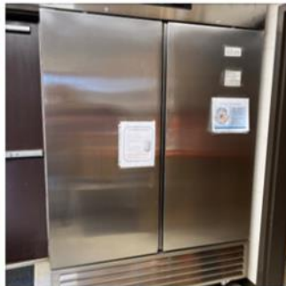
Replaced refrigerator in Lower Kitchen
